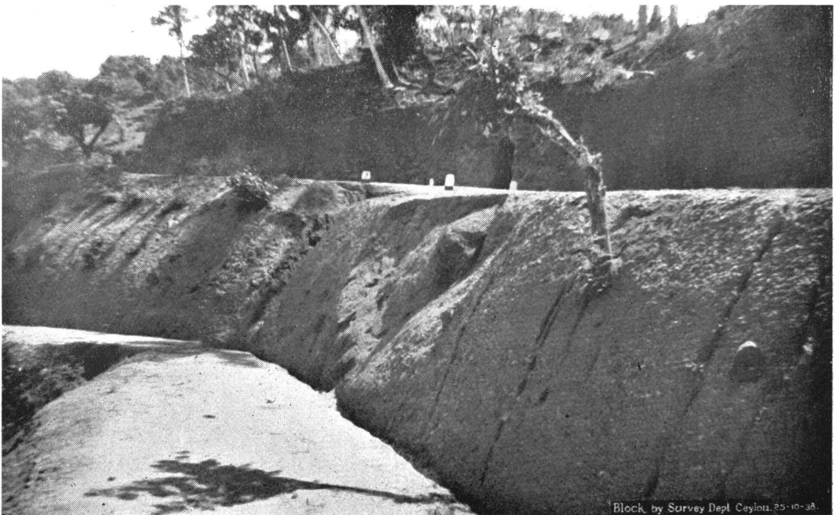
FIG. IV.—ROADSIDE BANK EROSION.
