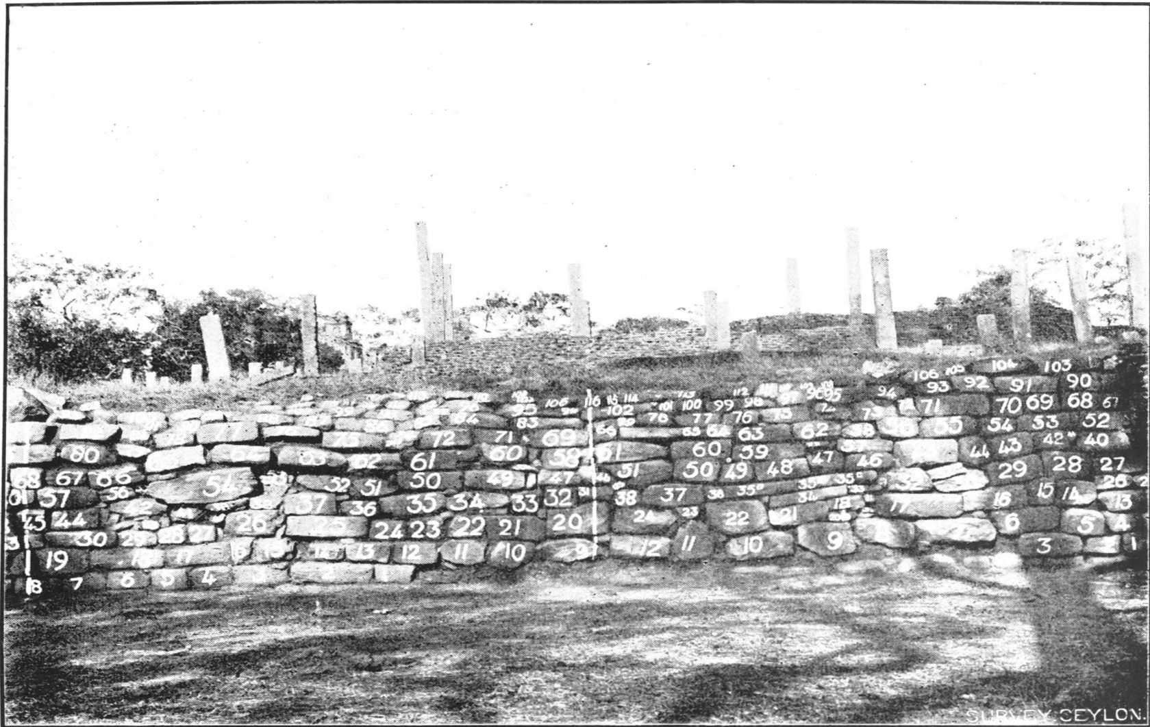
No. 1.—POLONNARUVA, RETAINING WALL OF THE QUADRANGLE, BEFORE CONSERVATION.
